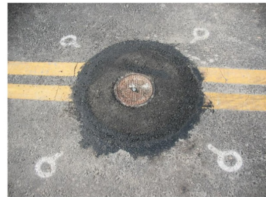
This is a monument well sometimes call a monument box. The 4 small circles are nails used to install the monument well.
