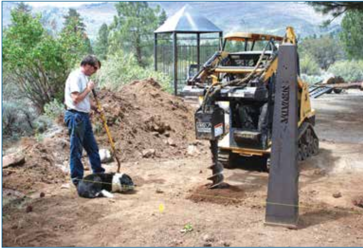
Casey Smith, owner of Black Bart Iron Works, and friend, preparing to place enclosure, May 8, 2014. Author's photo.
