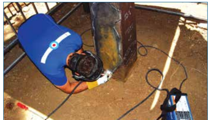
Paolo Cividino of Tutto Ferro applying first welds to patch, June 16, 2014. Author's photo.
