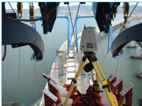
Laser scanning the single anchored suspension of the new SFOBB. Submitted by: Juan Barahona and Robert Dolan
