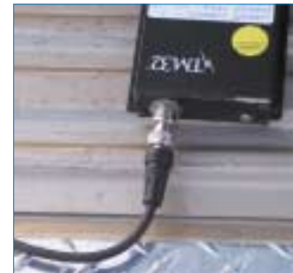
Fig 1b - One terminal on the antenna cable: much better.
