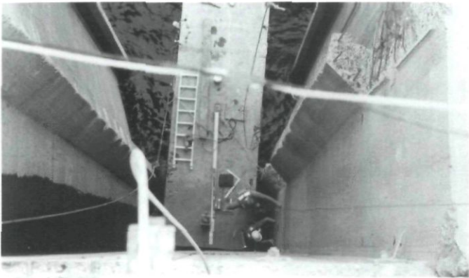
Iron worker Bud, and foreman Ray, of Fletcher General Construction, on a barge, setting control plates 70 feet below the top of the dam.
