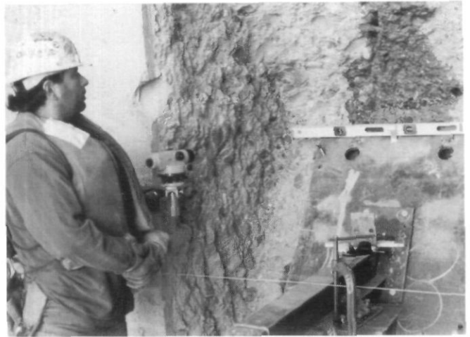
Ricky, an iron worker, admiring the placement of a drilling jig which is 70 feet below the top of the dam.
